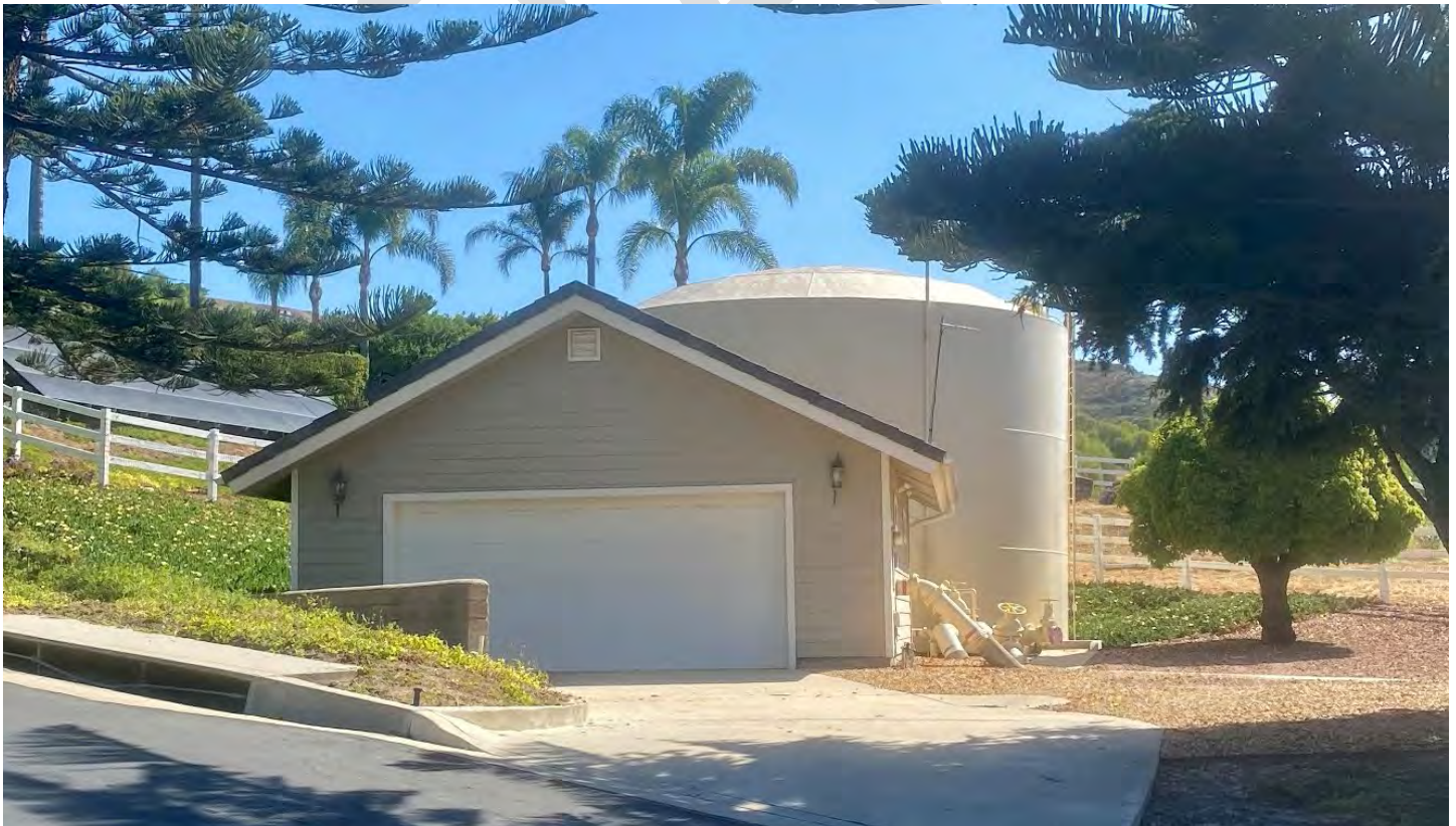
Non-Potable Tank and Pump Station
