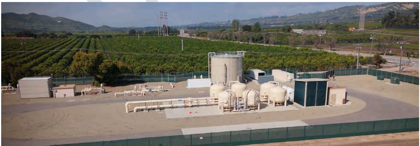
Conejo Wellfield Granular Activated Carbon (GAC) Water Treatment Plant
