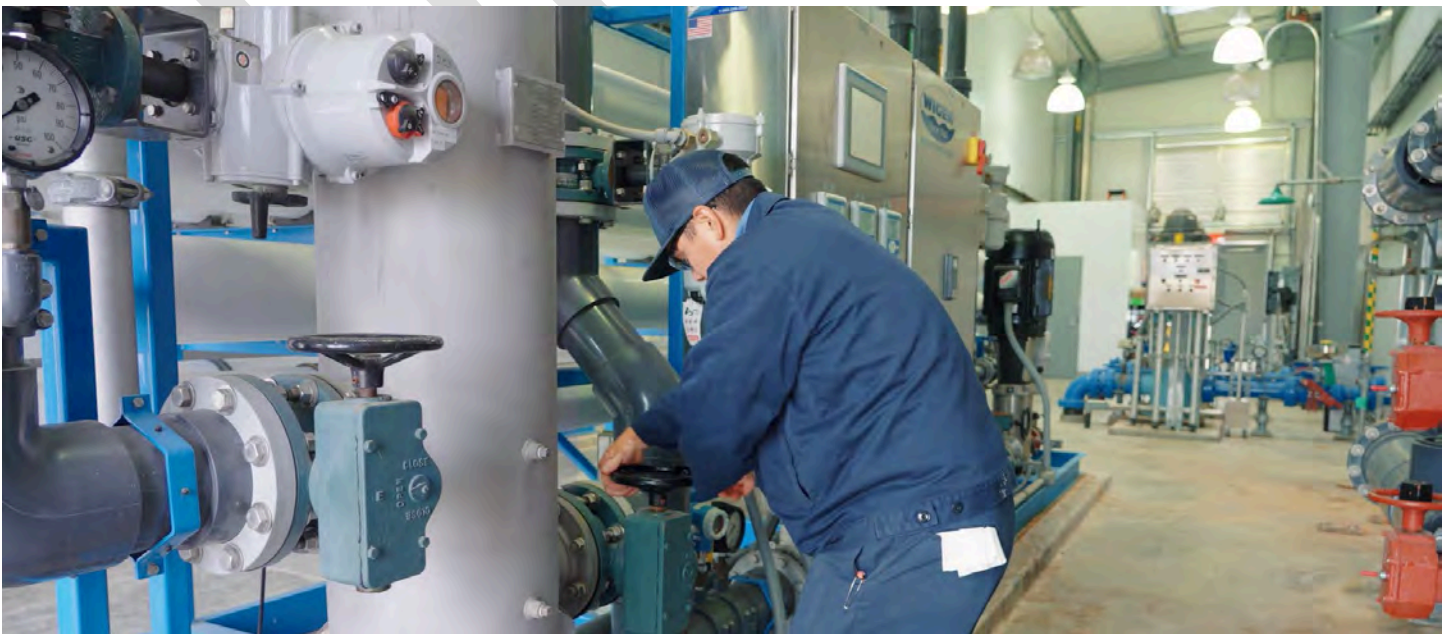
Round Mountain Water Treatment Plant Operations
