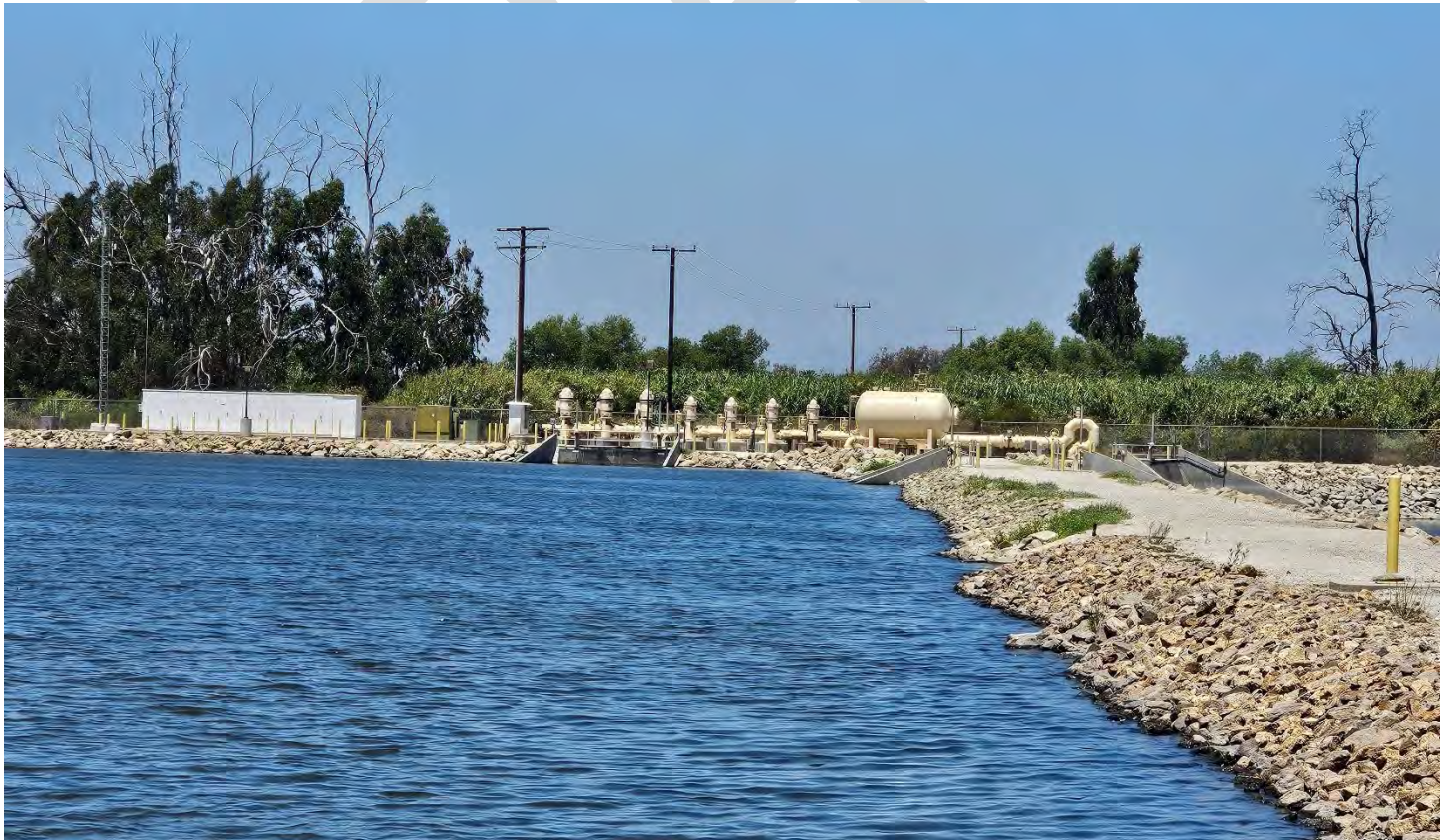
Non-Potable Storage Ponds & Pump Station
