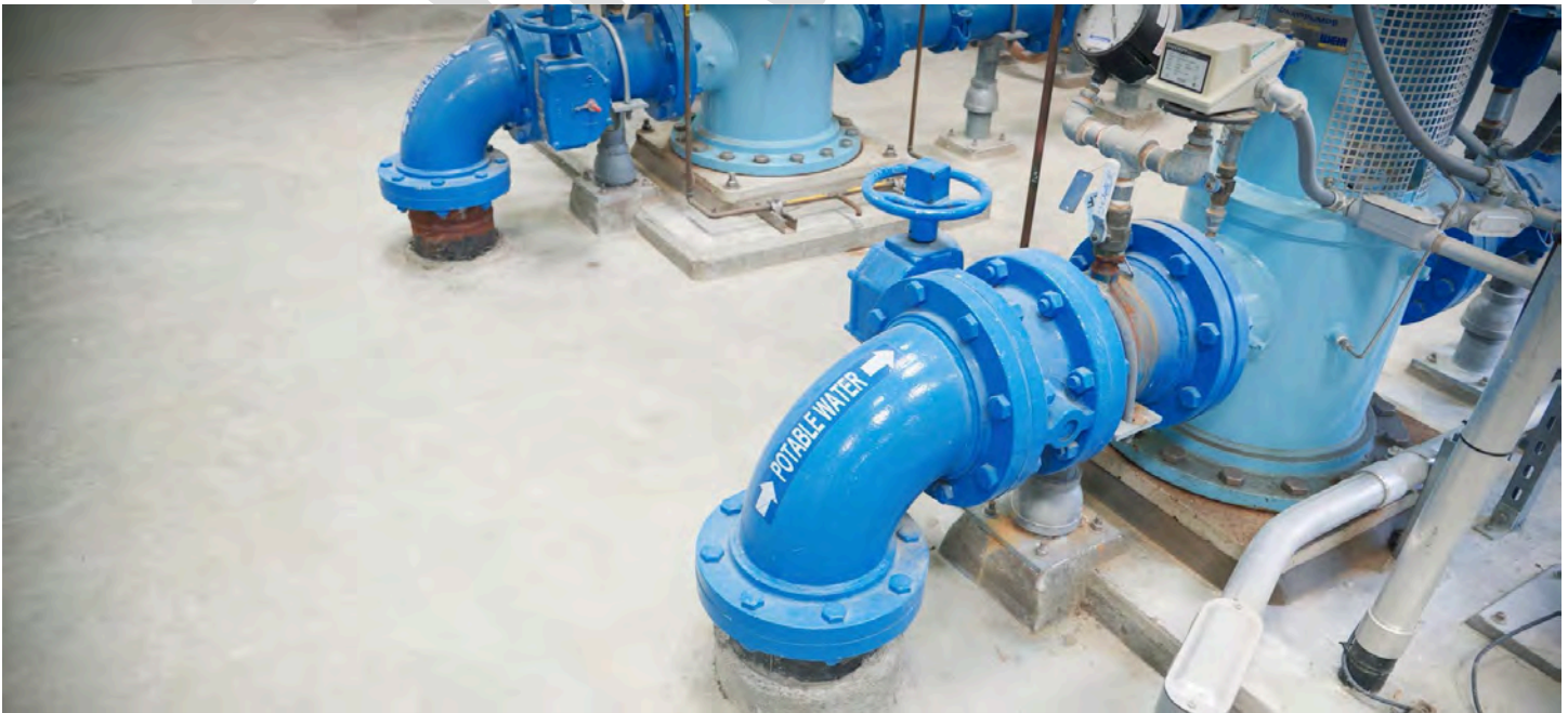
Potable Water Pumps
