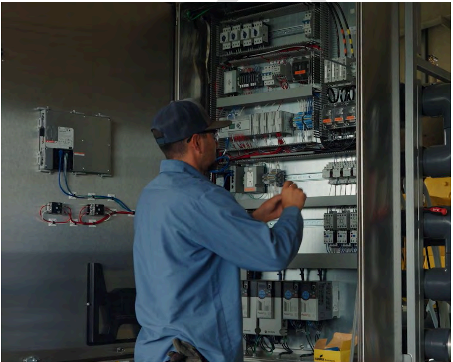
Supervisory Control and Data Acquisition (SCADA) Equipment
