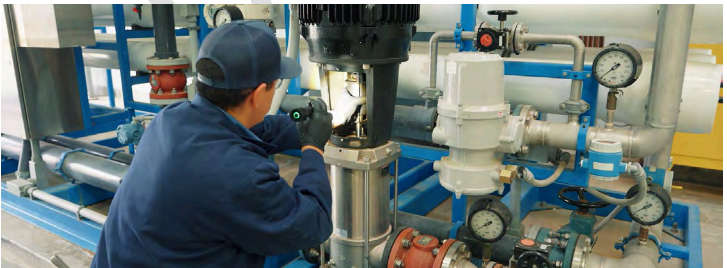
Pump Maintenance Performed by Camrosa Staff
