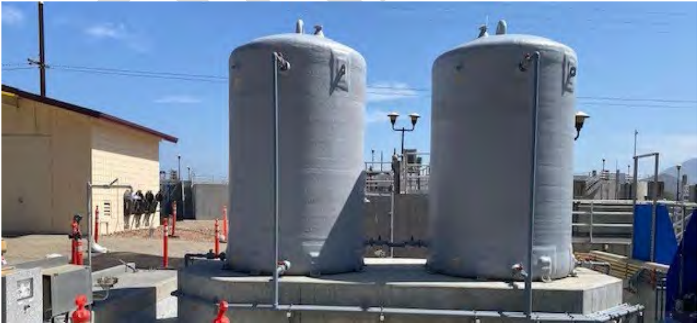
CWRF Chemical Feed
