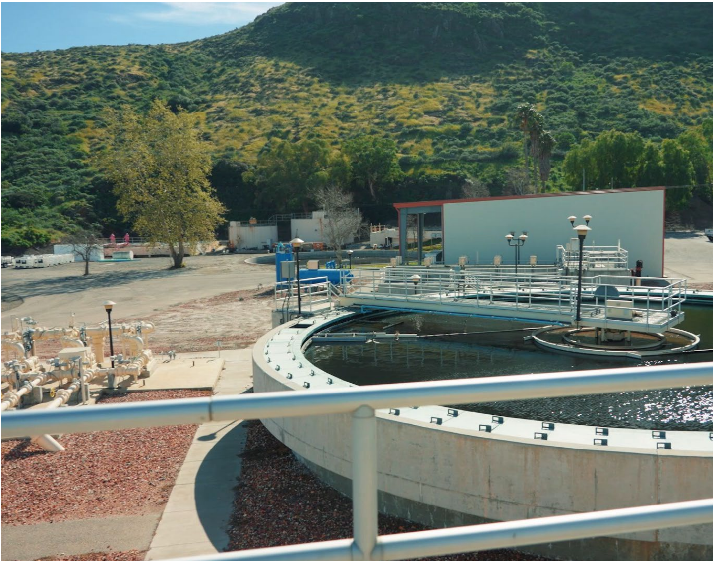
Clarifiers at the Camrosa Water Reclamation Facility (CWRF)
