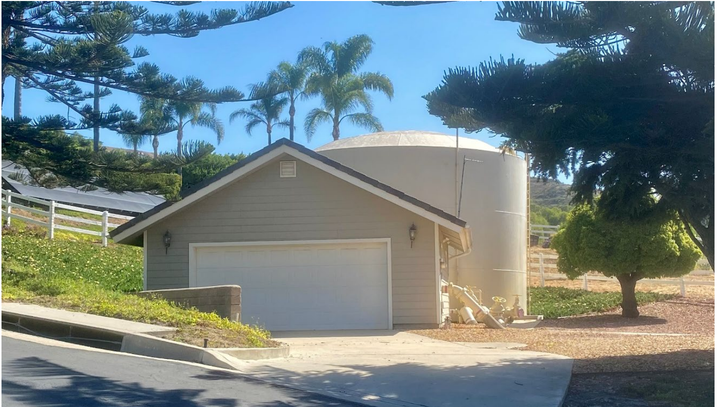
Non-Potable Tank and Pump Station
