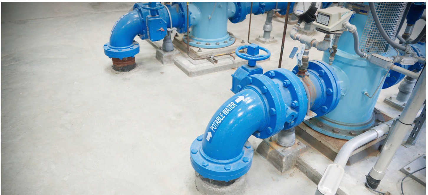
Potable Water Pumps
