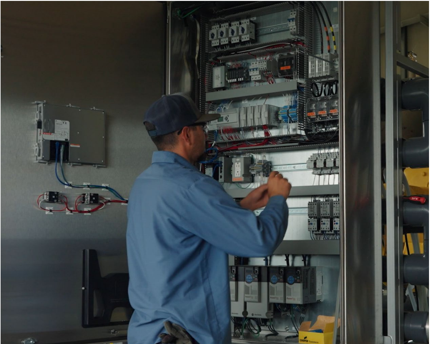
Supervisory Control and Data Acquisition (SCADA) Equipment
