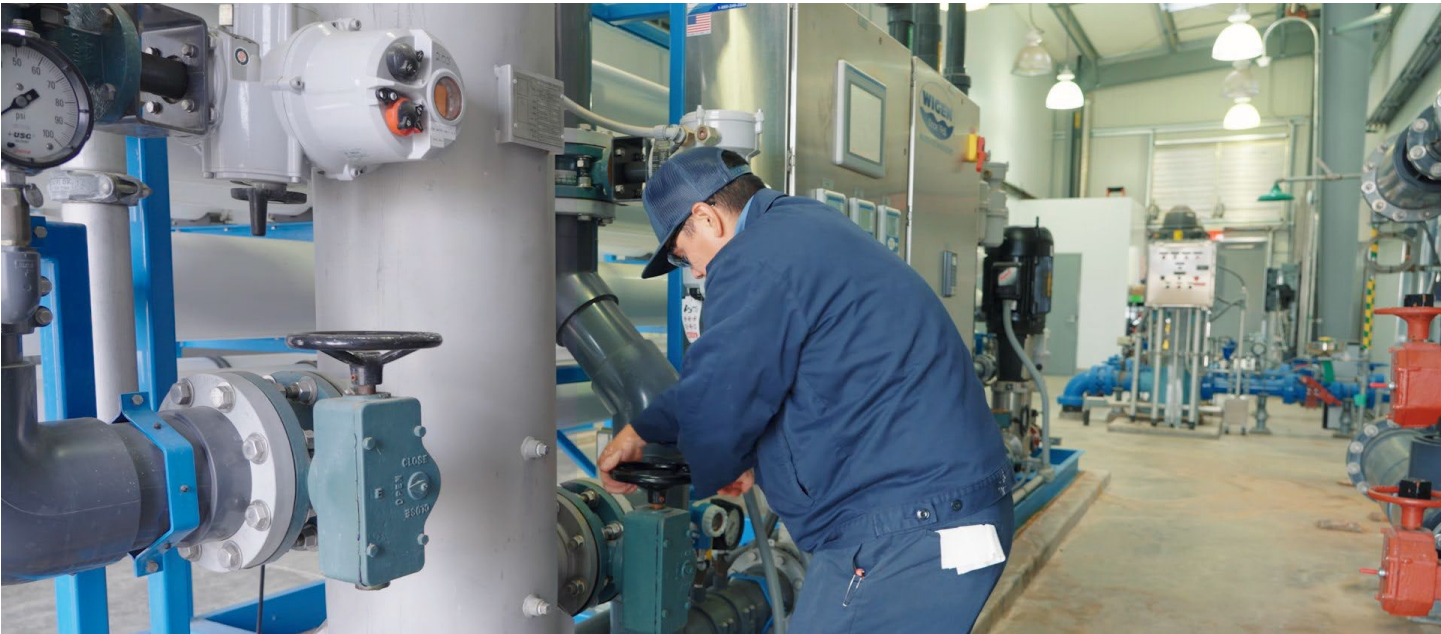
Round Mountain Water Treatment Plant Operations
