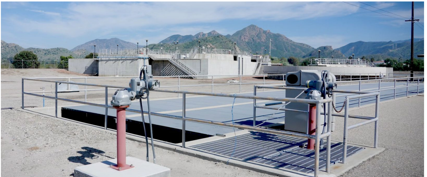
Sequential Chlorination Project at CWRW
