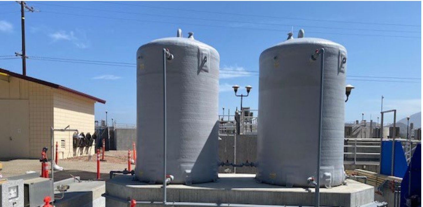
CWRF Chemical Feed
