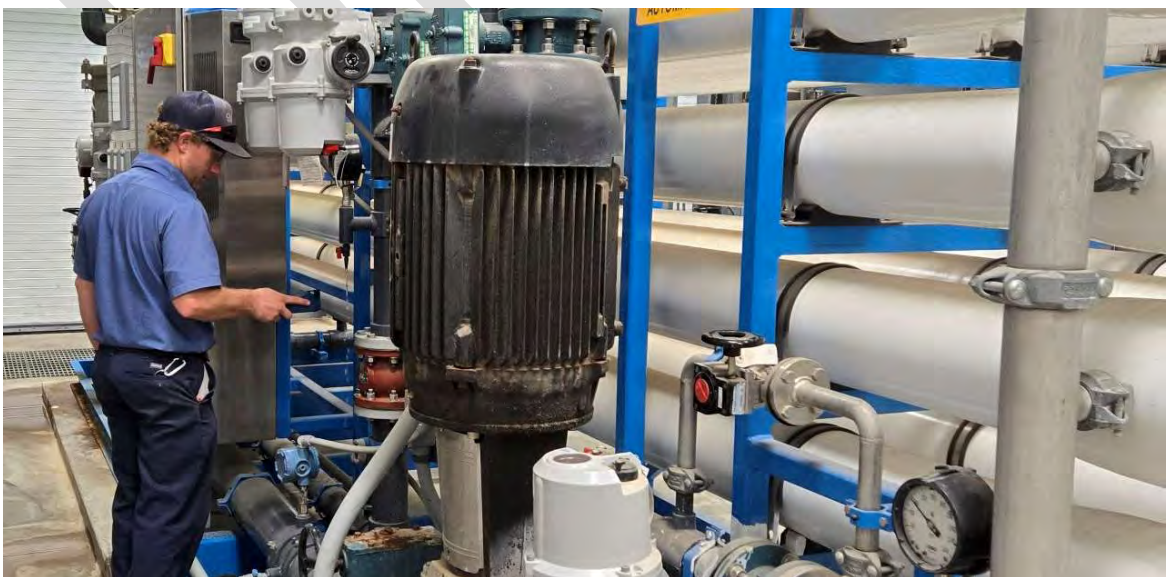
Round Mountain Reverse Osmosis (RO) Water Treatment Plant
