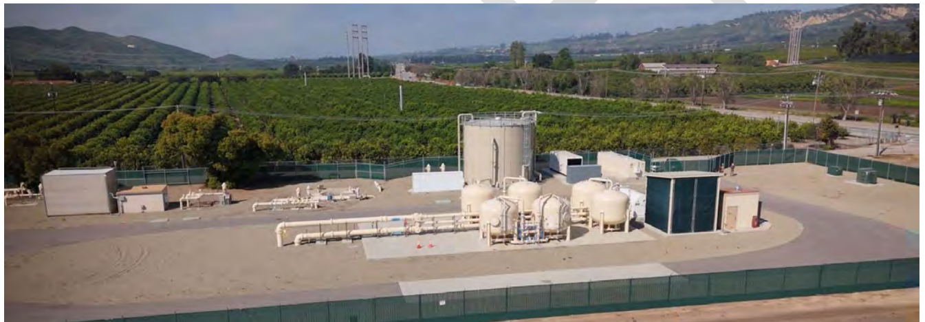
Conejo Wellfield and the Granular Activated Carbon (GAC) Water Treatment Plant
