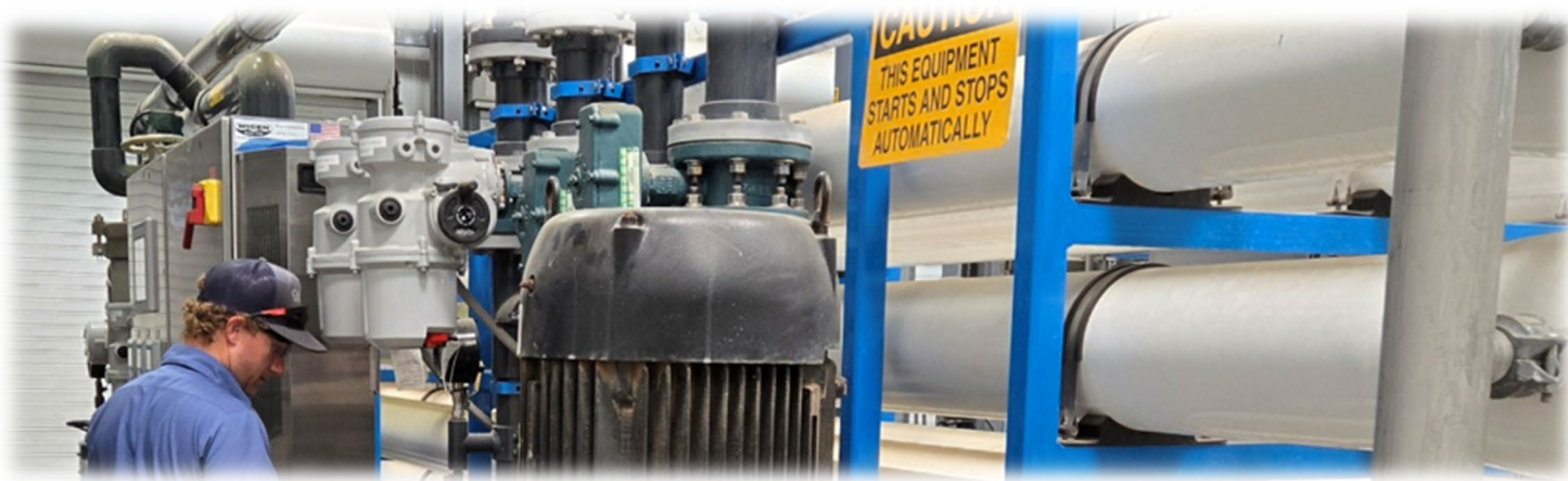
Round Mountain Reverse Osmosis (RO) Water Treatment Plant
