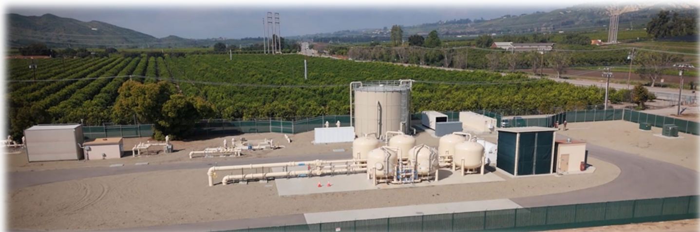
Conejo Wellfield and the Granular Activated Carbon (GAC) Water Treatment Plant
