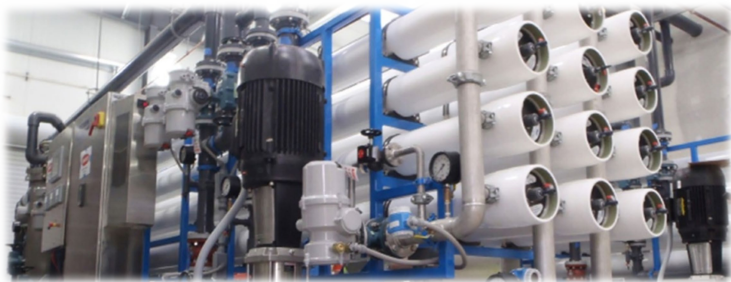
Round Mountain Reverse Osmosis (RO) Water Treatment Plant
